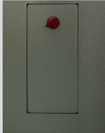
Figure 12: Pressure relief valve
